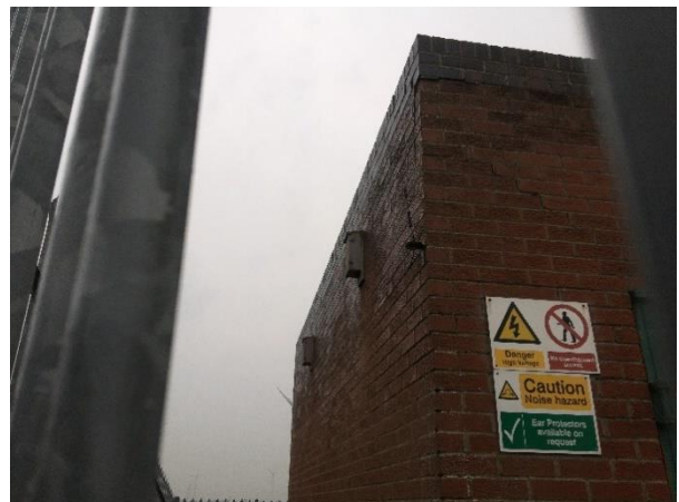
Photograph 10: TN1 Building with bat box and cracks in the building exterior. Cracks in the building have low bat roost potential.
